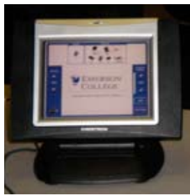
The Crestron Control Panel
